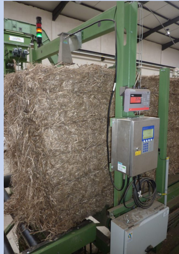
MicroPolar LB 567 system installed in France, measuring the moisture inside Hemp bales
