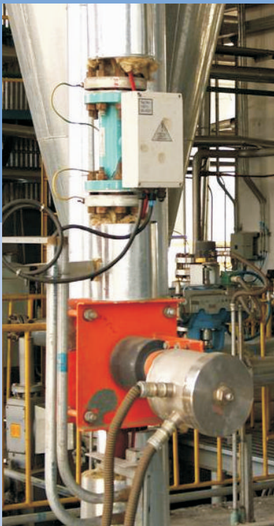
Installation on a pneumatic conveying line, with a DYNAvel velocity sensor.
